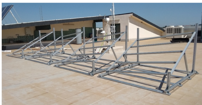
Fig. 8. Thermal solar field structure.
